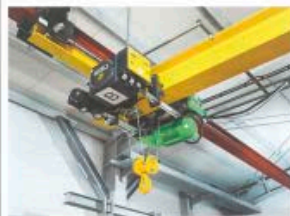
Stahl CraneSystems supplied all the crane technology, including explosion-protected wire rope hoists, suspension crane and carriage with explosion-protected travel motor and the control.
