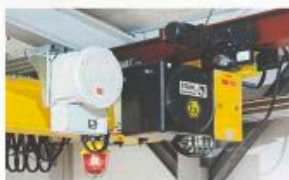
Here, meet the electric ATEX and IECEx equipment.
