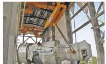
03 These turbines weigh more than 300 tonnes and are positioned with millimetre accuracy using rope winches with precise controls
