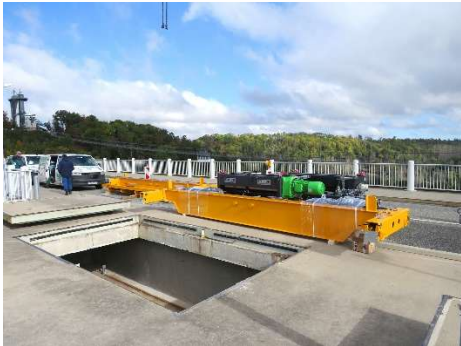
With an opening of only 2 m x 4 m, the hatch and the installation space are extremely narrow.
