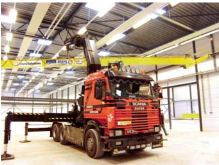
Picture 3: Assembly of single girder overhead travelling crane in the new building
